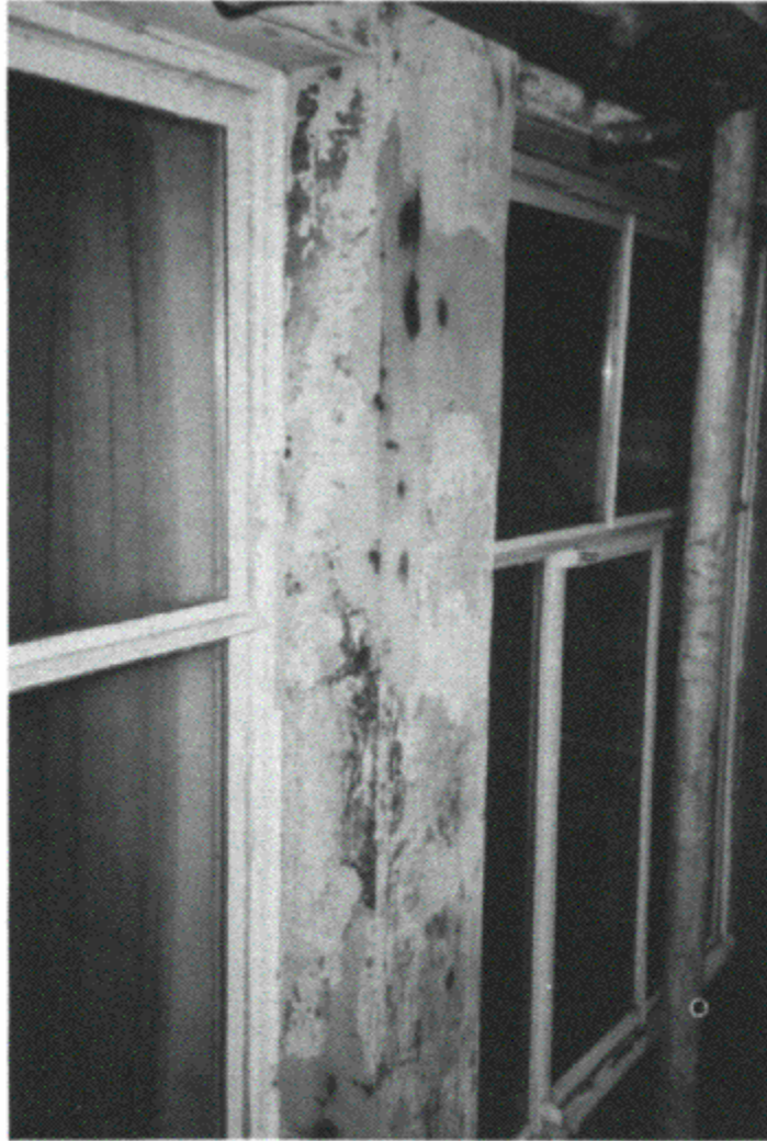
Figure 5.6 Incipient anodes formed around the edge of a poorly applied patch on a building exposed to salt.
