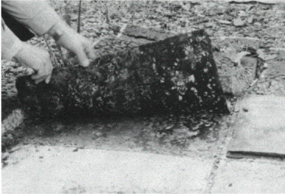
Figure 5.9 Waterproofing membranes can fail to bond, dissolve into the concrete under the application of the hot mix for the wearing course, or be punctured by the aggregates. Tighter specifications are now used in the UK to avoid systems prone to such failures. This photograph shows some of the membranes after testing at the Transport Research Laboratory.
