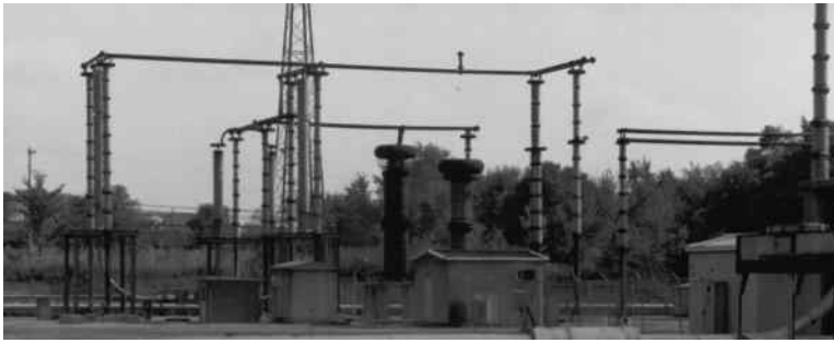
FIGURE 6.10 800 kV dc terminals of a converter station.
